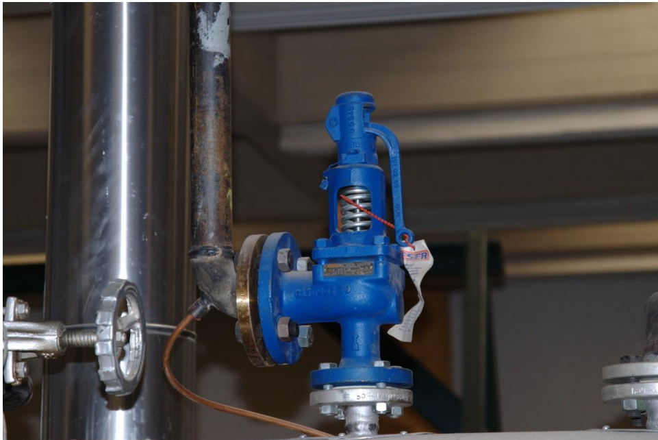
8.10. Rasteretni ventili (Blow down (vent) valves)
